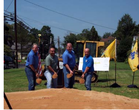
Freeholders Damminger, Chila, Director Sweeney and Harrison Committeeman Clowney break ground for Phase II improvements to 322 Richwood section.
